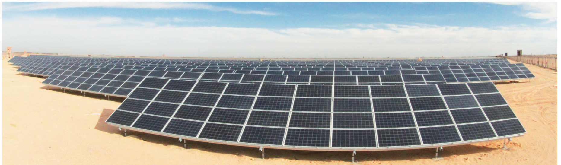
233 MW ground-mounted PV plant in Algeria - "Energy Oasis" in the Sahara Desert
