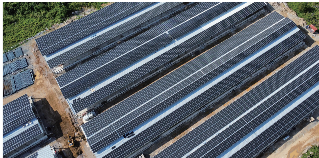
The integration of animal husbandry and Photovoltaics Project in Tiandeng county
